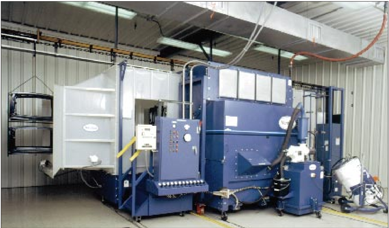
The Nordson booth has a translucent polypropylene canopy that diffuses ambient light and is nonconductive.
